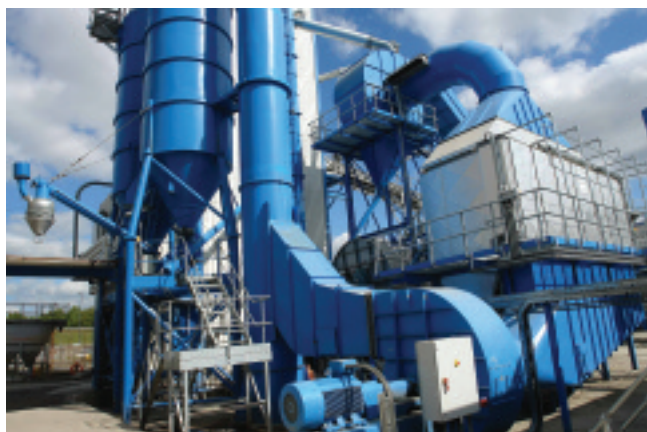
View of dust collector, fan and exhaust stack
