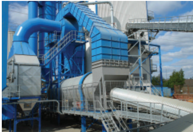
The 2.8m diameter x 10m long fully lagged and clad aggregate dryer
