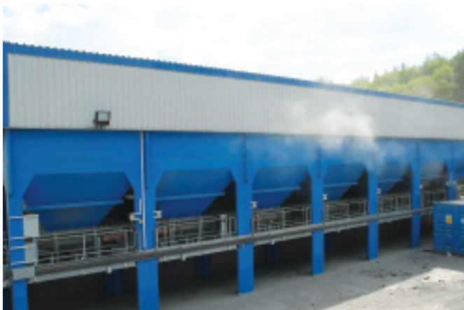
Seven-compartment covered cold-feed unit
