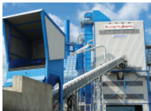
RAP system showing feed hopper and inclined conveyor to mixer level
