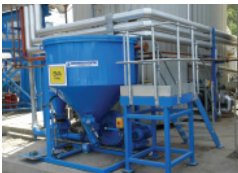
Granulate additive system with blower
