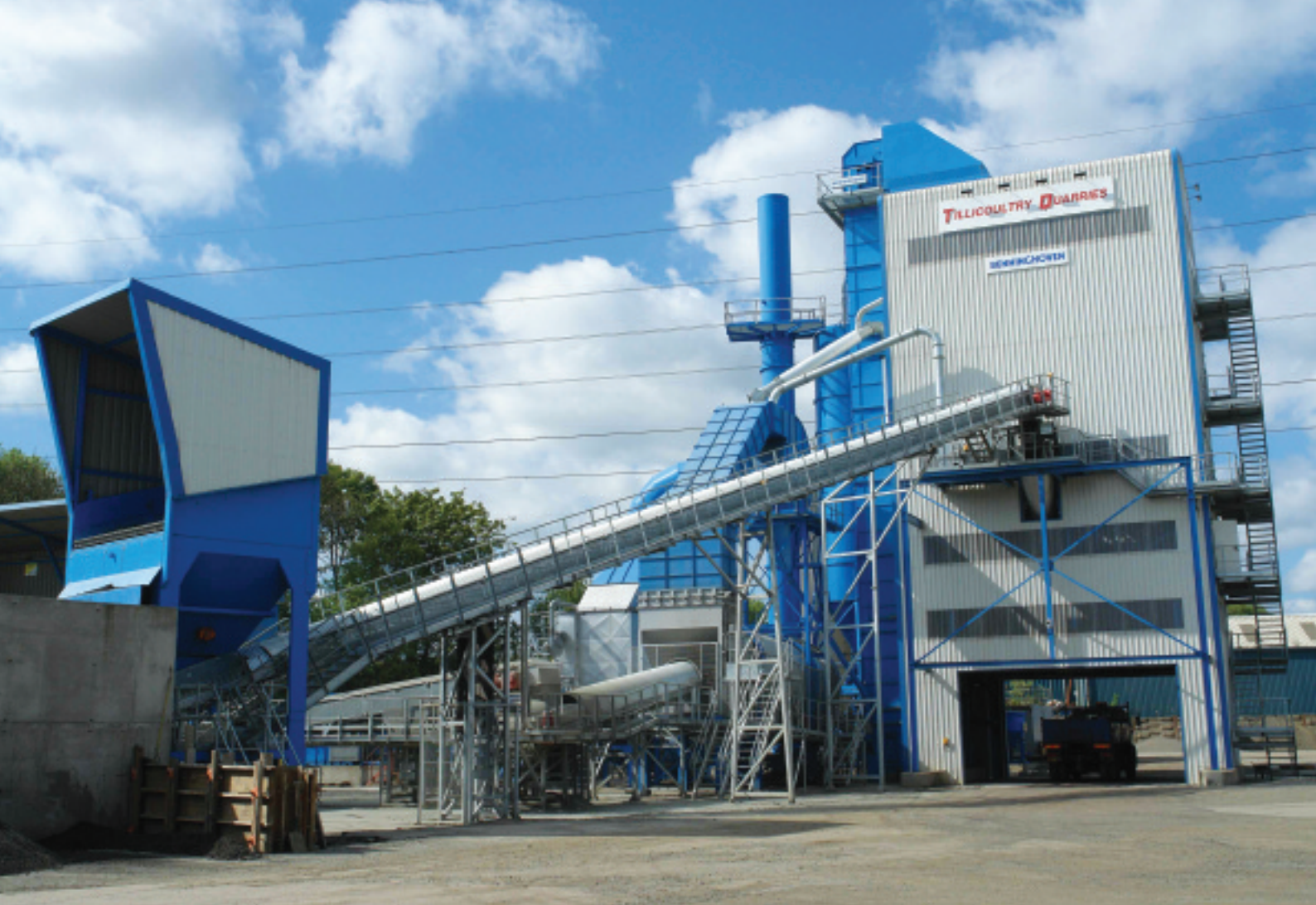
New Benninghoven model BA4000 asphalt plant at Tillicoultry Quarries' Clydebridge site
