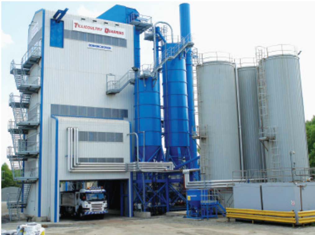
Fully sheeted plant tower with imported and reclaimed filler silos
