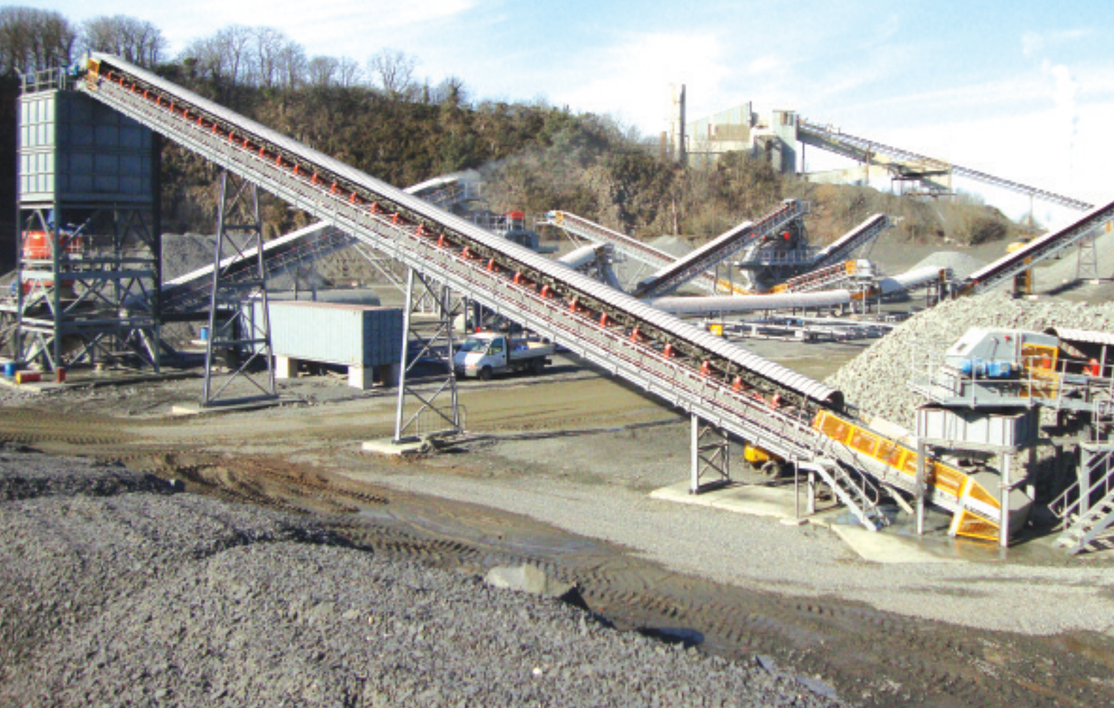
The new secondary crushing and screening circuit at Hillhouse Quarry with the existing main crusher building/screenhouse visible on the skyline
