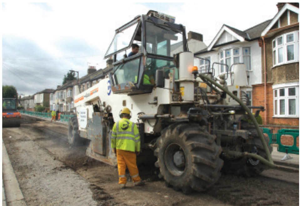
By adopting in-situ recycling Newham BC have saved around £80,000 and more than 9 tonnes of CO 2 emissions
