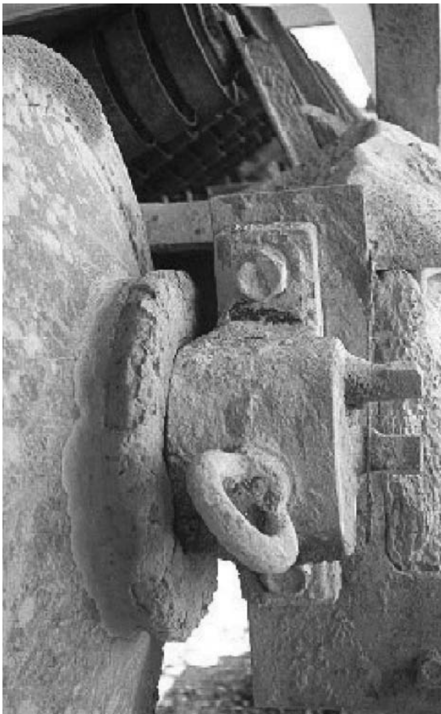
Application: Fertilizer and potash. Still in work after more than 30 years in an aggressive environment.
