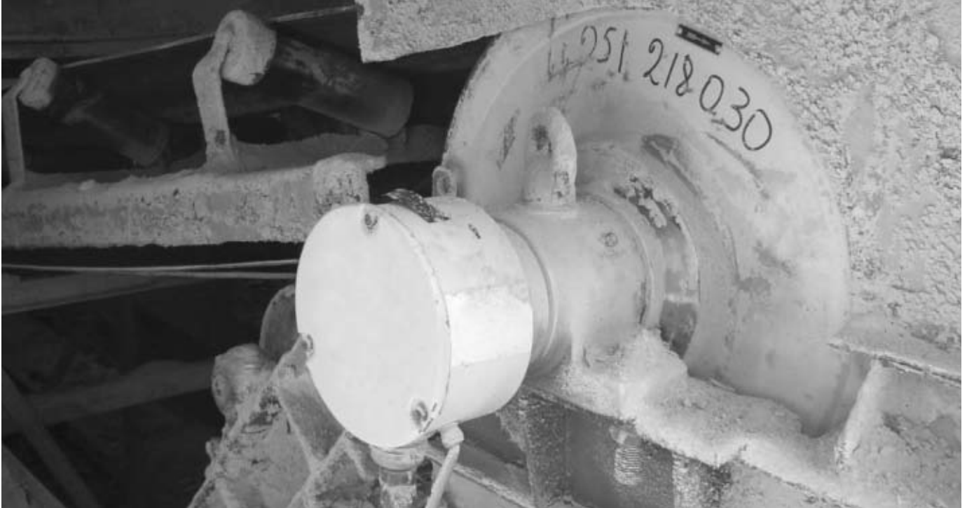
Aggressive & abrasive potash application located in the desert. Features: Re-greasable IP66/67 seals, insulation class H motor, NO maintenance and operating through Frequency Converter.
