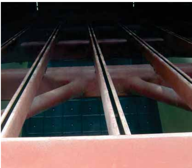
LS-SR rails on construction screen
