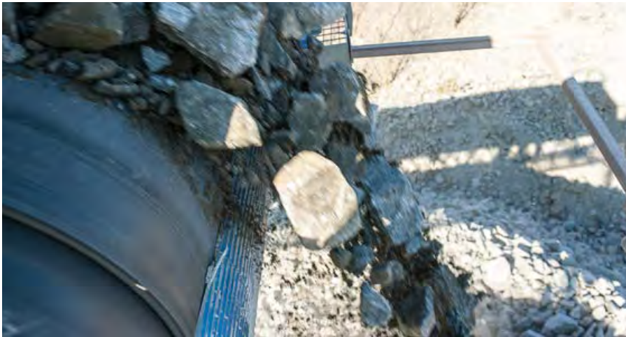
In the majority of cases, the primary belt cleaner is positioned on the head pulley, which is where the material leaves the belt.
